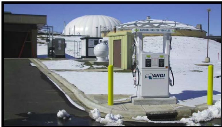
Figure 6: BioCNG installation at Janesville, WI WWTP (BioCNG, 2012)
