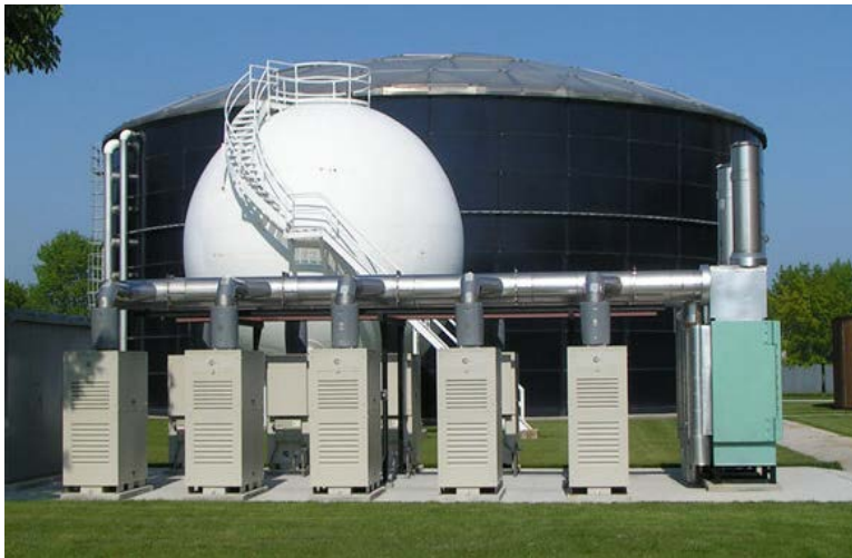
Figure 5: Microturbine Installation at the Sheboygan Regional WWTP
