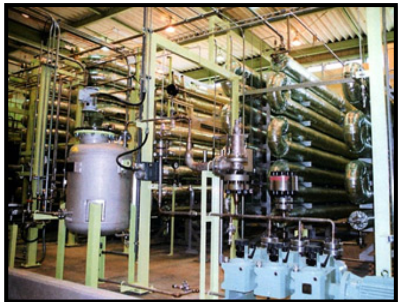
Figure 2: Supercritical Water Oxidation Facility in Cork, Ireland
